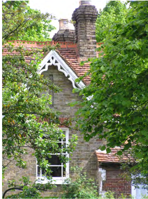
Picture 2.65 Decorative timber bargeboards, and clay ridge tiles on a property along Stanmore Hill
