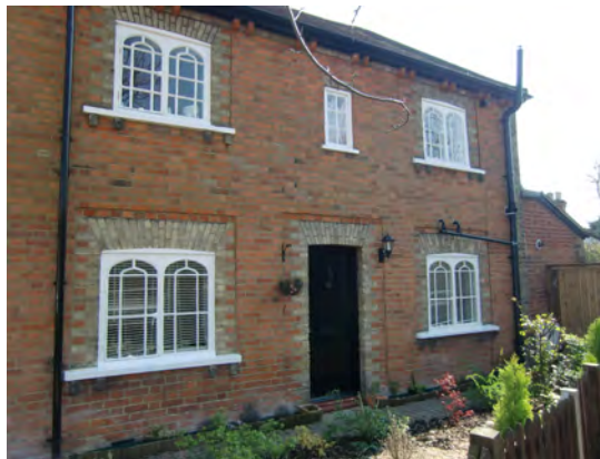
Picture 2.57 No. 12 Green Lane Cottages and its decorative brick quoins and brick surrounds to windows
