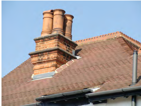
Picture 2.60 Prominent chimney with clay chimney pot, decorative ridge tiles and tile banding detail, Green Lane
